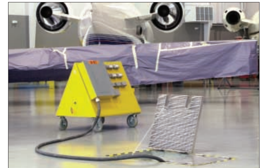
Buried tunnels bring compressed air, electrical power and computer/telephone wiring to the aircraft and workstations via the "power pits." Each aircraft utilizes a junction cart (seen here in yellow) that provides electrical and air manifolds for multiple technician use.
