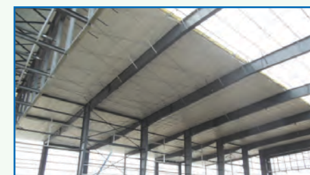
Roofing for the south hangar of the building is progressing through the Nebraska winds.
