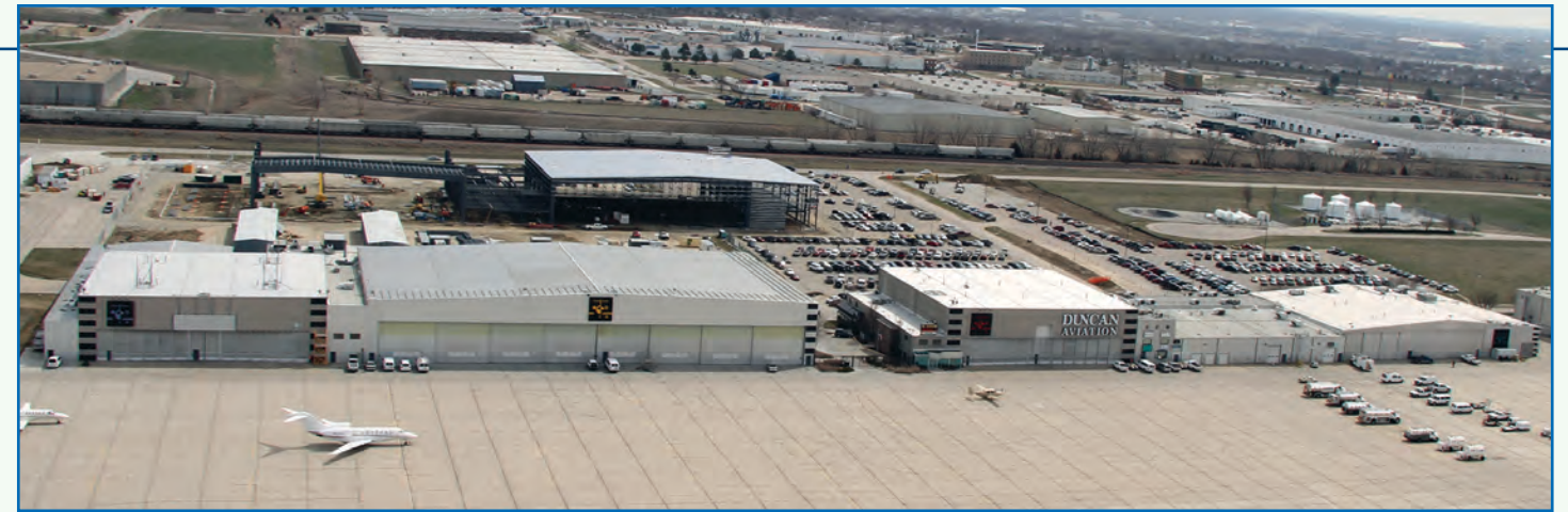
April 2013 - Steel for the north hangar going up. The overall dimensions of the building are 630' by 200'. The hangar will stand 46' tall at the eave and approximately 52' at the peak.
