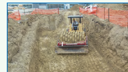
Compacting the trench that holds the electrical service. Fly ash was used to achieve the proper moisture content in the soil.
