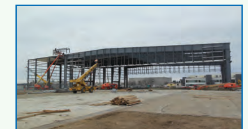
An overall view of the south hangar taking shape on the east side of the building. The jobsite was organized to accommodate 45 semi truck loads of steel that arrived March 18-27.
